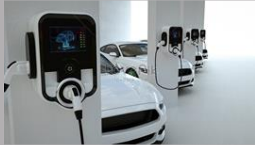
shared EV chargers
